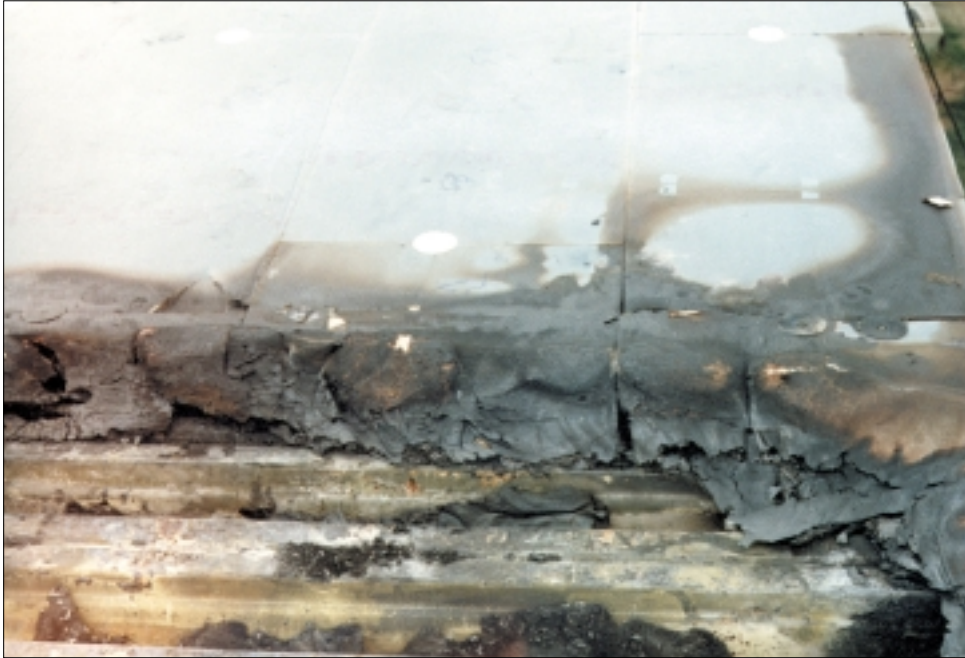
Figure 7: Roof after test - CFC blown foam
