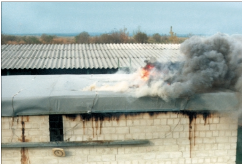
Figure 3: Roof during fire test - CFC blown foam
